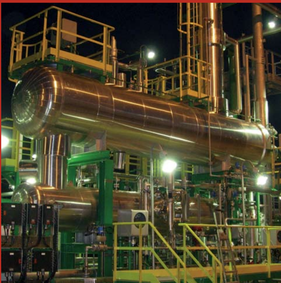
Gas dehydration plant with TEG technology
